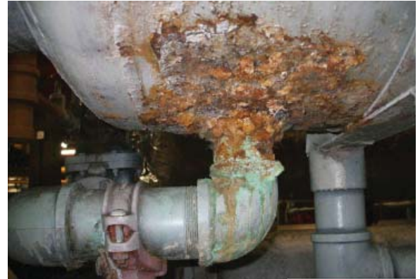
Inefficient and bulky tank-type heaters are prone to corrosion and leaking.
