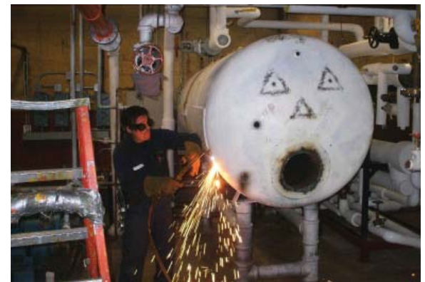
Armed with a cutting torch and safety goggles, Paul DeCanio dismantles this bulky beast to make way for sleek, compact and energy efficient Armstrong Flo-Rite-Temp® instantaneous hot water heater.
