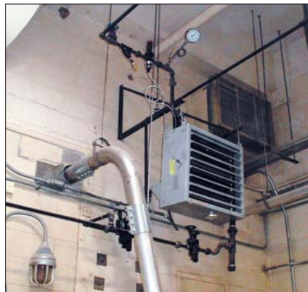
A permanently mounted steam heater in the sifting area of a Chicago, IL flour mill. Photo courtesy of Armstrong Intl. Inc.
