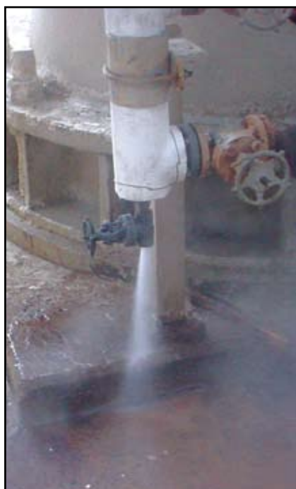
FIGURE 2. Open valve discharging to atmosphere
